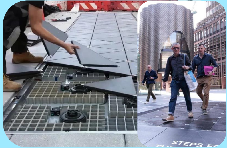
KINETIC mats - energy Harvesting
